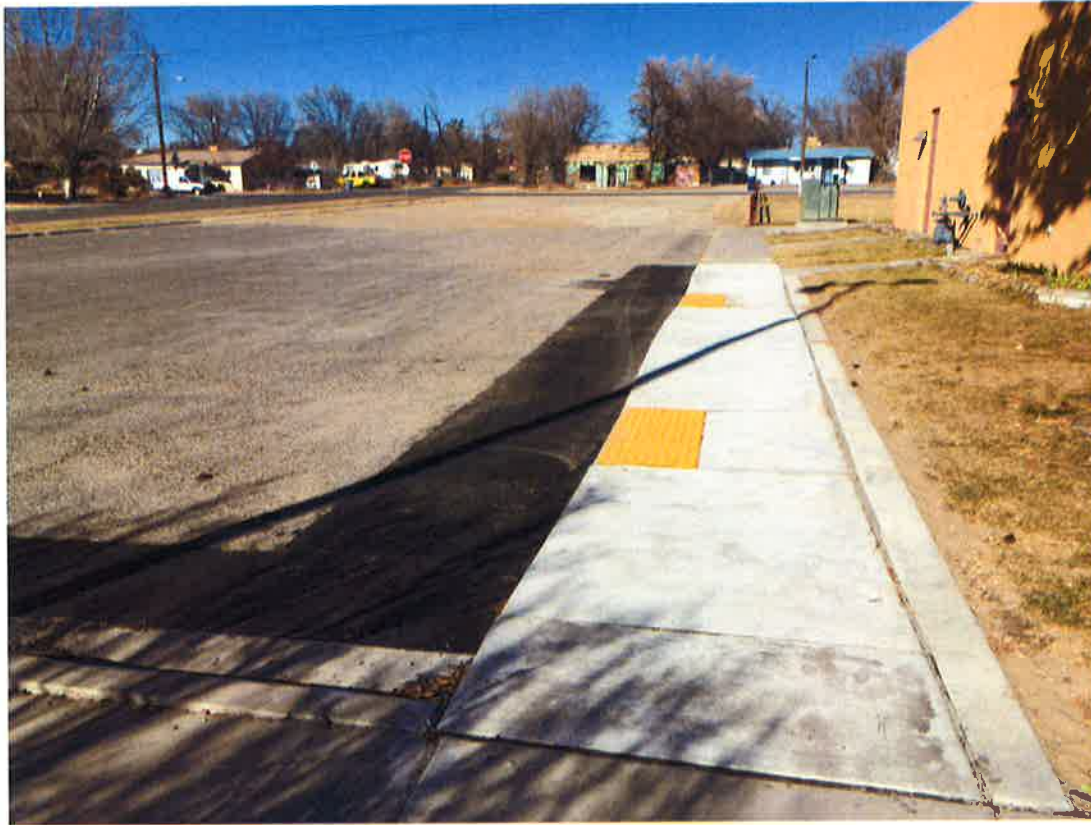
Cultural Center/Fitness Center: New ADA Curb Ramps for New ADA Spaces (awaiting signage and striping) by City Forces 2017.
