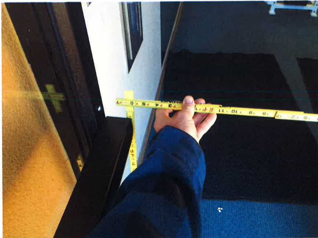
Cultural Center/Fitness Center: Fitness Center Door – Panic bar replaced to project < 4" into clear width. Completed by contractor 2017.
